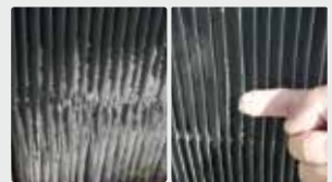
Cooling tower grids
