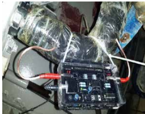
Vulcan 5000 was installed on the water inlet of the water recycling room.
