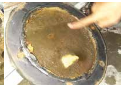
Inside of heat exchanger. Condenser end plate had lost all scale that was there previously. (Light spot at bottom is reflected light.)
