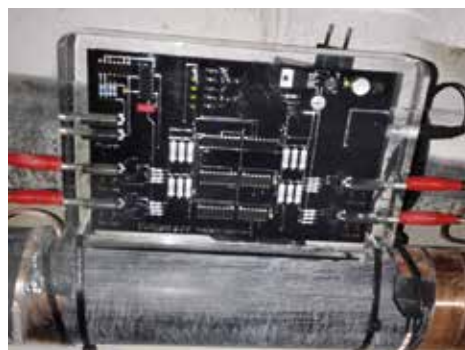
Vulcan S25 installed in on the heating system for 132 apartments
