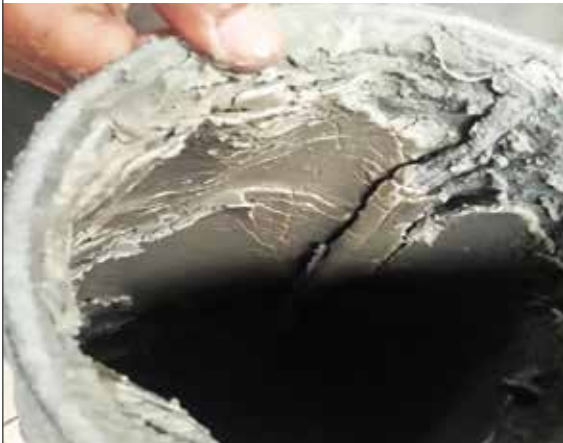
Without Vulcan, the filter was quickly stuck by scale deposits, and it had to be changed every 48 hours.
