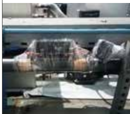
February 07 : Vulcan 5000 was installed before the Machine 1.
