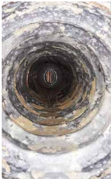
The scale deposits were easily removed with a water gun.
