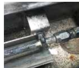
May 10 : The Machine 2 without Vulcan, the scale and bacteria are still on the walls and deposit in the water bottom.
