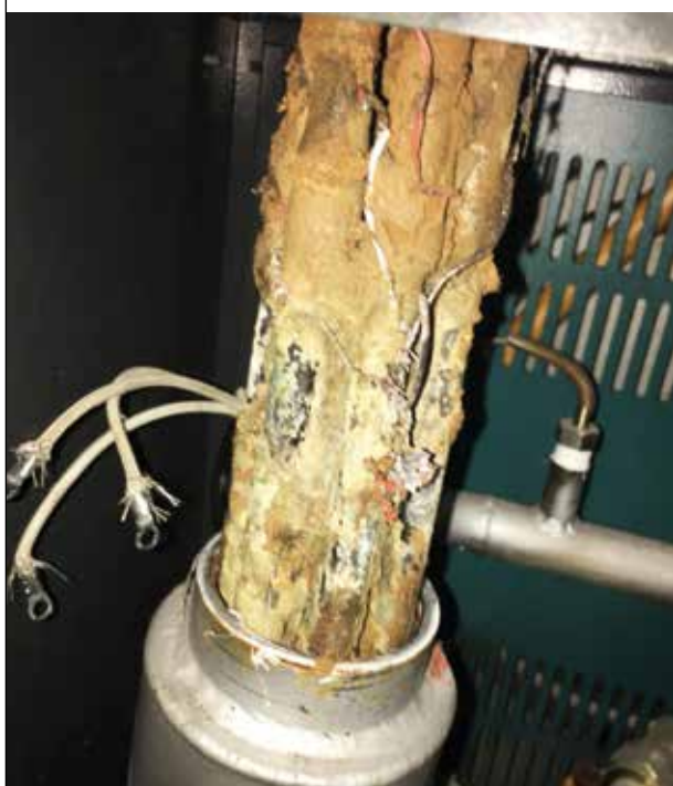
Untreated heat exchanger for 3 years.
