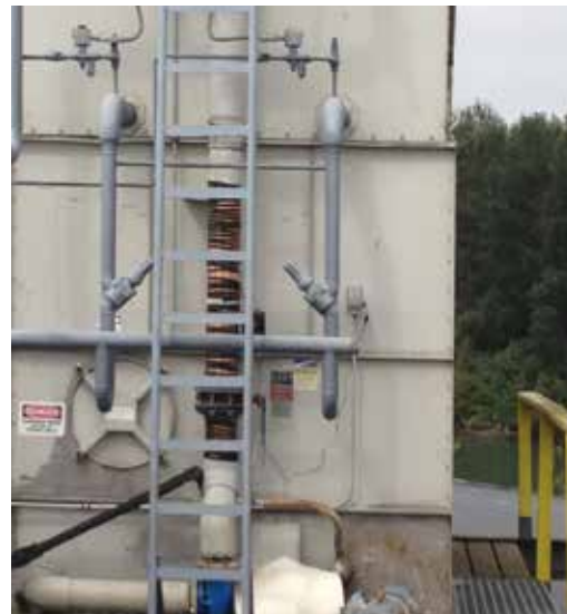
Vulcan S100 installed outside
