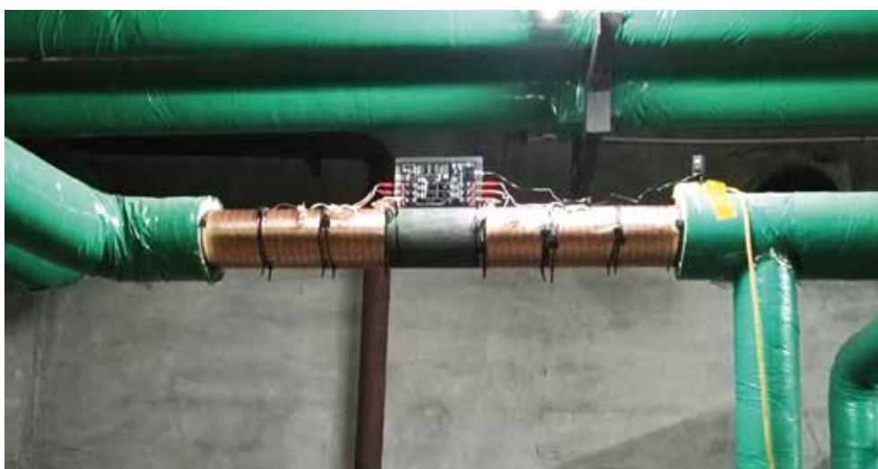
Vulcan S100 was installed on the main circulation water supply, which is from the municipal water.
