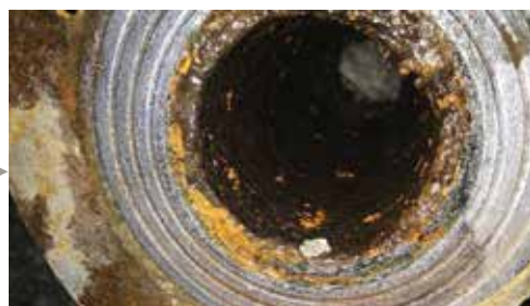
After Vulcan was installed for 3 months, the outer rust had been fallen off completely.
