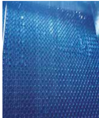
This photo was taken of the inside of CT-1.
