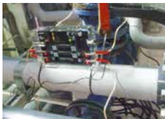
Vulcan S25 installed on the main water line
