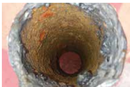
Before Vulcan was installed, the pipe was scaled and rusty.
