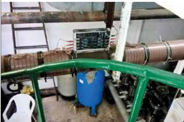
Two Vulcan S100 were installed.
