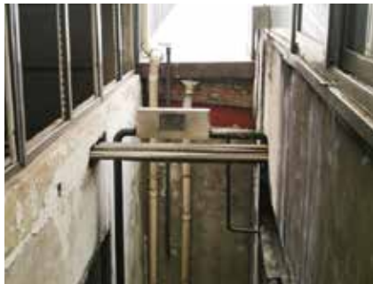
Vulcan S25 outdoor installation
