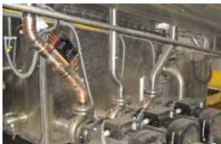
Vulcan S100 units installed on the produce cleaning system
