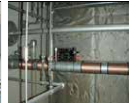
Used for the cooling towers C
