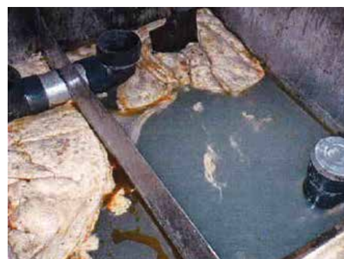
3 months after installation - grease is more consistent and less cluttering
