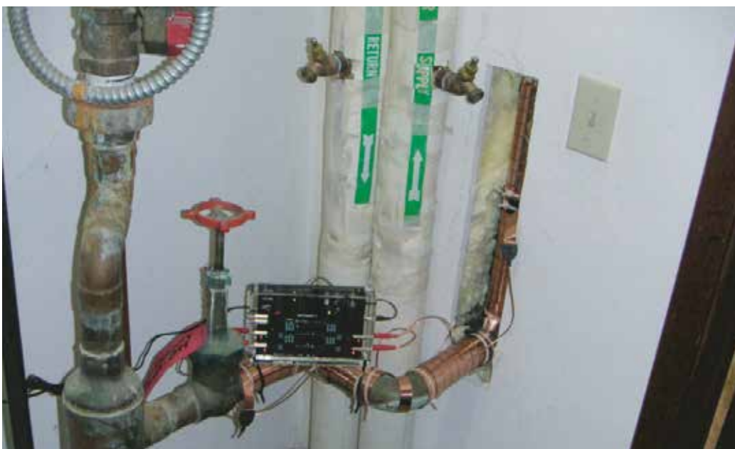
Vulcan S25 installed in Building E at the Health Center
