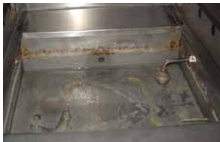
Before Vulcan installation - hard scale build up in the pan area
