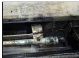
February 07 : Visual observation of the Machine 1 before Vulcan was installed. The wall and the nozzles have scale and bacteria.
