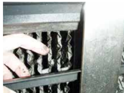
After Vulcan was installed for 5 months: the scale can be removed easily with a finger.
