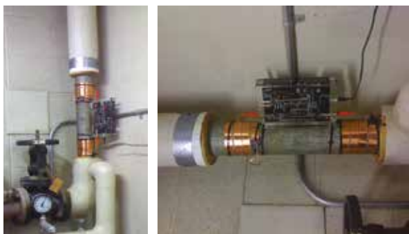
Installation of Vulcan Descaler for the entire buildings water supply in the Roosevelt school
