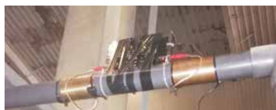
S10 was installed before the reverse osmosis membrane.
