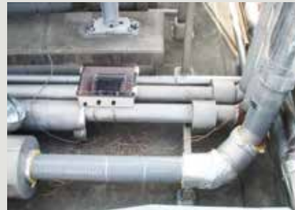
Vulcan S100 installation
