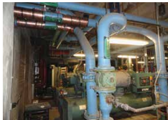
Vulcan S100 units installed on the double chiller
