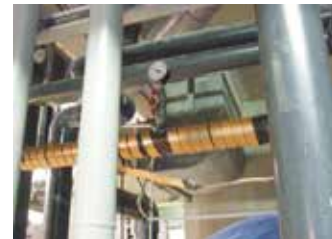
Vulcan S25 impulse cables
