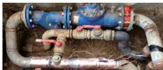
Vulcan S25 installed in the Alcoa Aliminum factory in France
