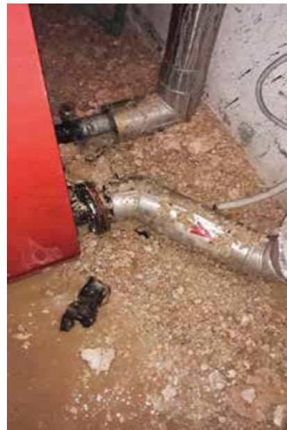
The scale deposits were drained out of the boiler with ZERO chemical.
