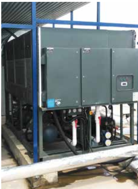
main air-conditioning system
