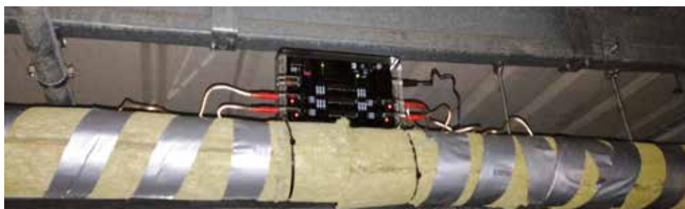
Vulcan S25 unit installed with insulation re-wrapped over the pipes and impulse cables
