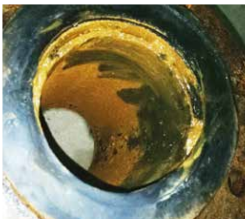
Scale can be easily wiped off, and the pipe shows the smooth wall
