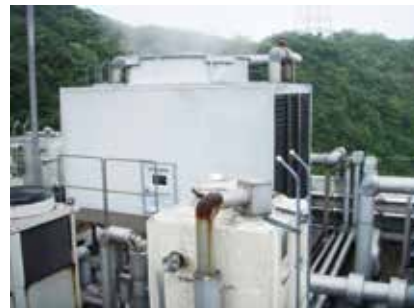
The cooling tower roof of medicine factory
