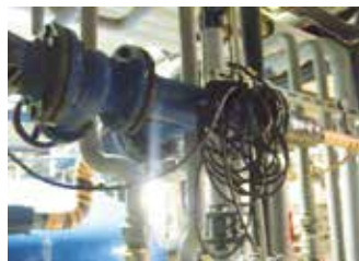
Vulcan S25 impulse cables
