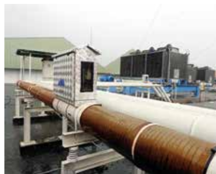
Vulcan S500 was located inside aluminum box and installed on a cooling tower main pipe in Supermal Karawaci.
