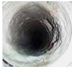
2 weeks after Vulcan was installed, scale had been softer and fallen out.
