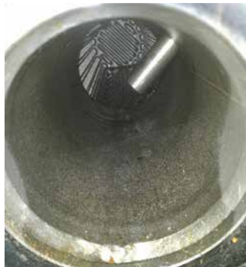
After 3 months – with Vulcan treatment. Up to now the installed pipe line needed no cleaning.
