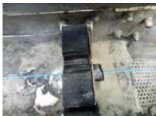
May 10 : The Machine 2 without Vulcan, the scale deposits on walls and coils.
